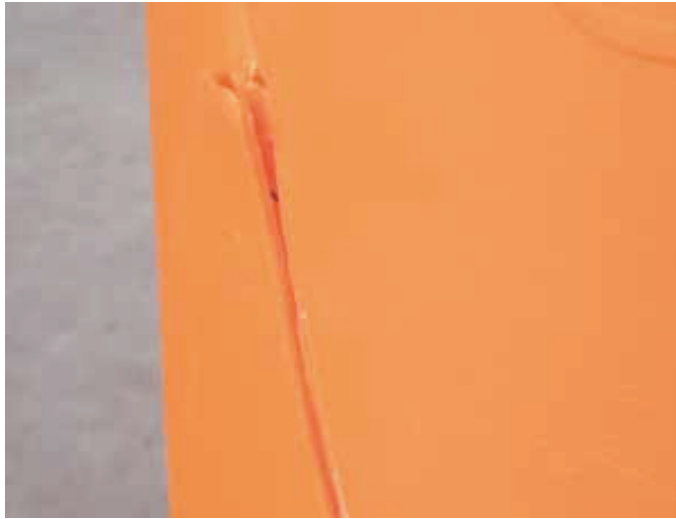
Figure 7a Cuts & Gouges (level 2) – Repairable
